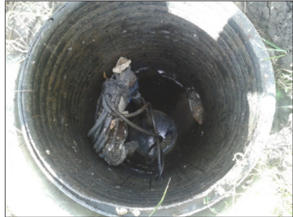
Figure 7. Visible degradation of internal manhole elements
