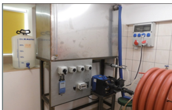
Figure 11. Fundamentals of Technology Department Laboratory – control panel of the rotating biological contactor with bi-directional longitudinal flow
